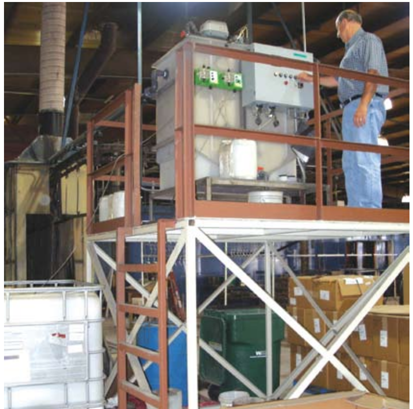
The heart of the system is this control and clarifier module, which automatically monitors and replenishes the pretreatment solution to maintain proper operating conditions.
